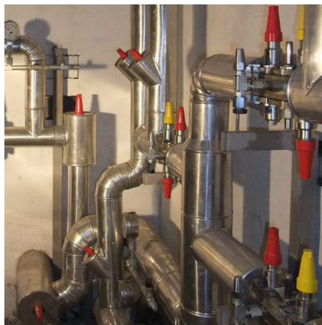
Fig 2: The use of ICF Flexline™ valve stations on the distribution lines of evaporators in storage rooms
