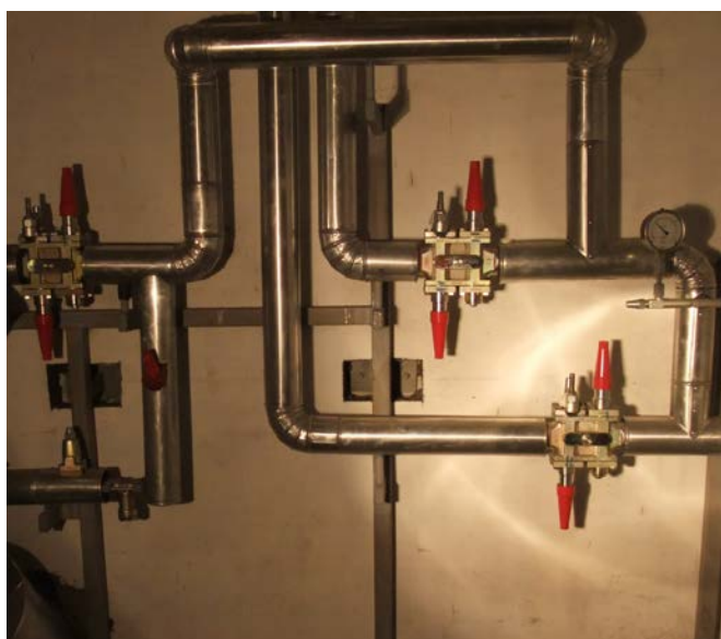
Fig 4: ICF Flexline™ valve stations on defrost lines
