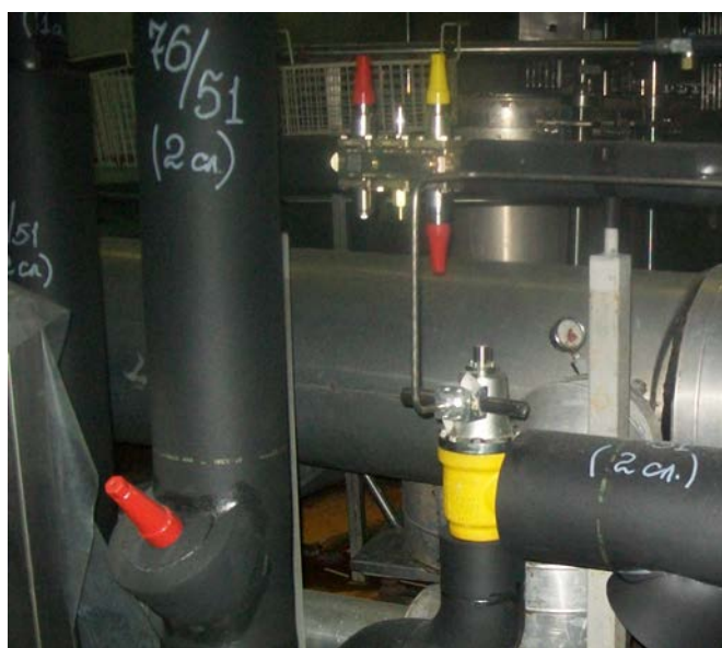
Fig 3: ICF valve stations fitted on evaporator defrosting lines
